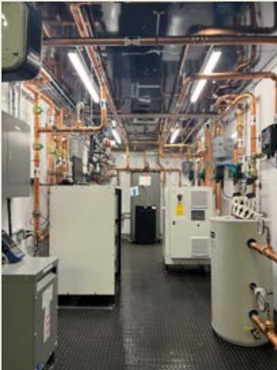
Inside of Trailer
